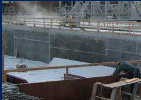
Waste water treatment plant, Canada
