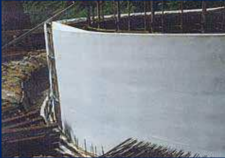
Water tank*, Grossglattback, Germany
